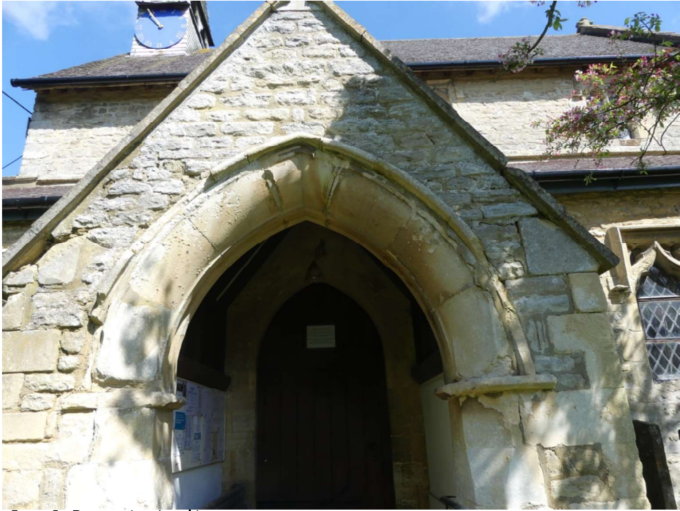
Figure 5 - Decay to hoodmould
