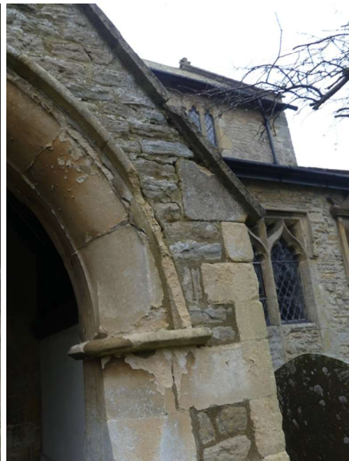
Figure 7 – Decay to the east of the arch
