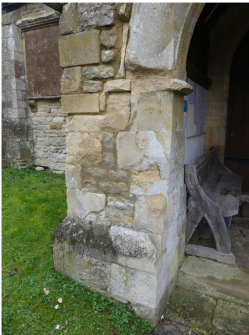
Figure 6 – Decay to stonework to west jamb
